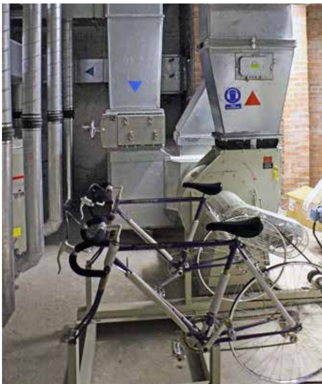
Ventilation and air filtration plant room with mounted bicycles for use in the event of power failure. Virtually unscathed since Nick Catford's photographs of 2001
